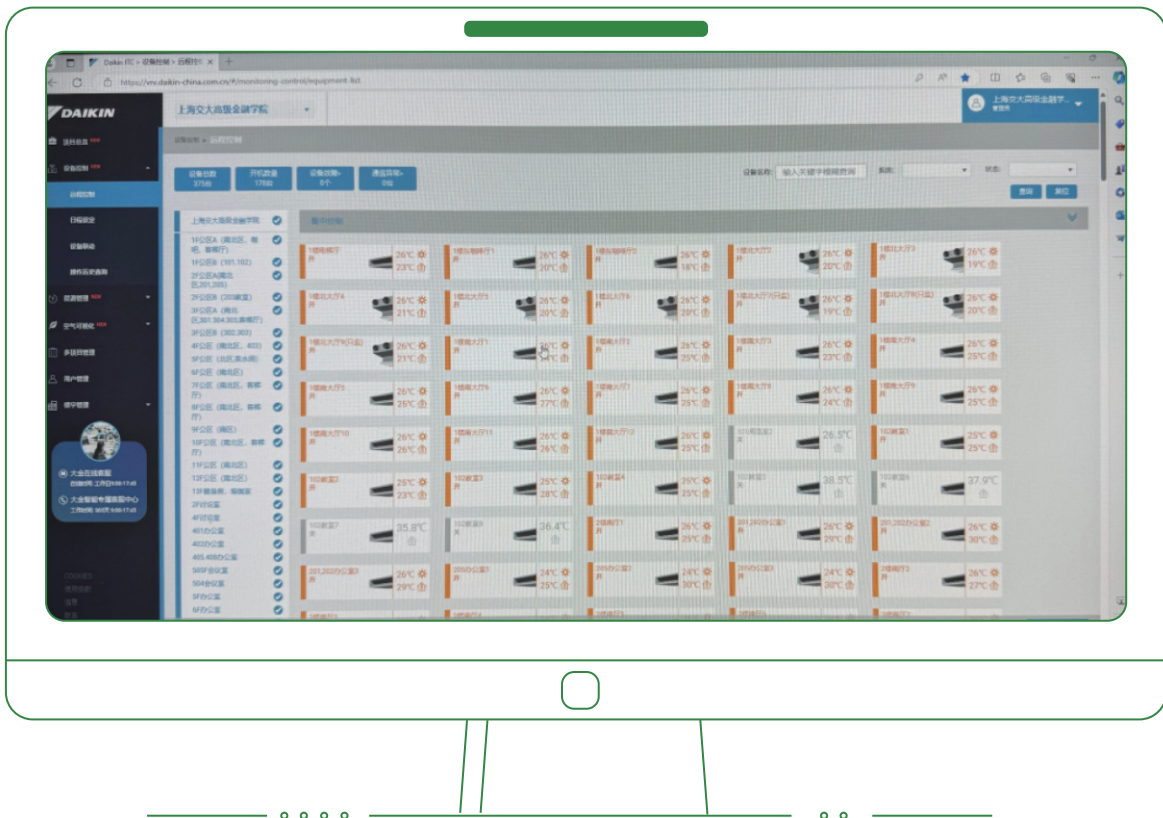
Figure: Control System Display Panel of SAIF
